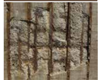
Steel Rods corrosion
