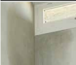
Internal Wall Dampness
