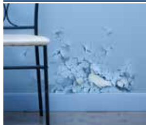
Paint peeling off
