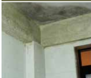
Leakage from ceiling
